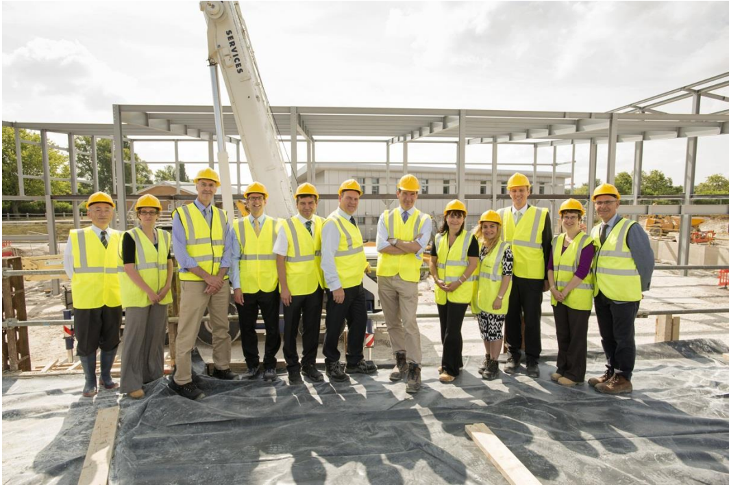
Photo taken at the building site area of I14 beamline and the Materials Characterisation Facility L/R: Yasuo Takemitsu (JEOL), Julia Parker, Diamond beamline scientist (I14), Trevor Rayment, Diamond's Physical Sciences Director, Paul Collier, Johnson Matthey Research Fellow, Dogan Ozkaya, Johnson Matthey, Peter Ash, Technology Manager: Advanced Characterisation, Johnson Matthey Technology Centre, Andrew Harrison, CEO of Diamond Light Source, Elizabeth Rowsell, Director, Johnson Matthey Technology Centre, Sarah Karimi (JEOL), Andrew Richards, Diamond's Legal Manager, Elizabeth Shotton Diamond's Head of Industrial Liaison, Paul Barrett, Diamond's Commercial Manager
